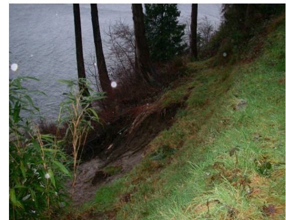
✘ Recent slope failure in Davis Bay/Selma Park after heavy rains.
