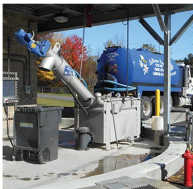
Photo 2: Septage Receiving Station and Screening Removal
