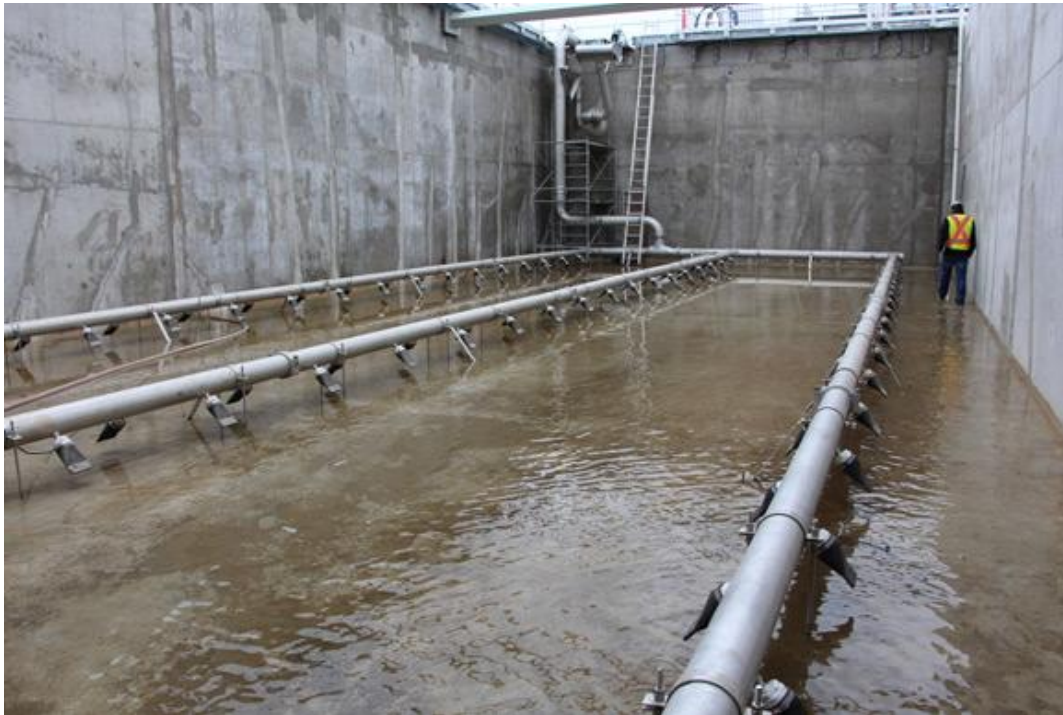
Photo 1: Aeration Mixing System
