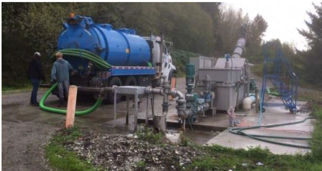
Photo 8-1 Road Septage Receiving Facility
