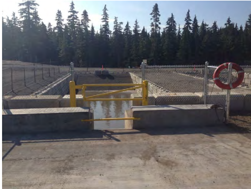
Photo 8-2 Septage Dewatering Facility at Forceman Ridge Landfill, RDKS
